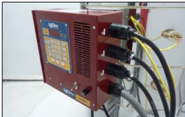
All element jumper cords installed:
