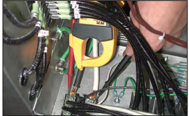
Checking voltage at the power terminal block.
